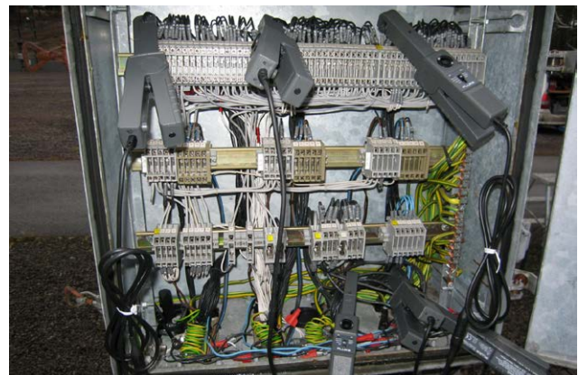
Figure 3 Control cabinet with current clamps
