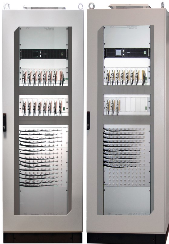
Fig. 9: Partial Discharge Acquisition Racks (PDMAR)
