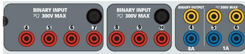
Figure 250 Binary Inputs 4 to 10 and Binary Outputs 4 to 6
