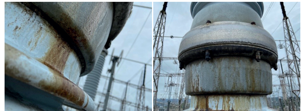
Figure 6: CVT-2 as found during visual inspection
